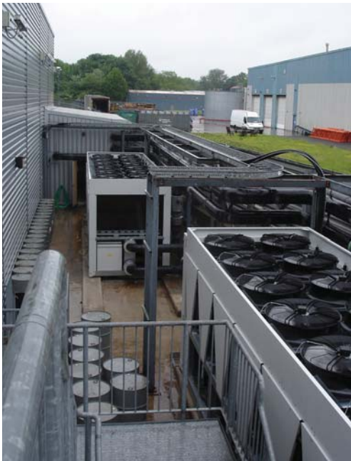
DeltaChill™ FreeCool chillers providing free-cooling to indoor units in a Manchester data centre
